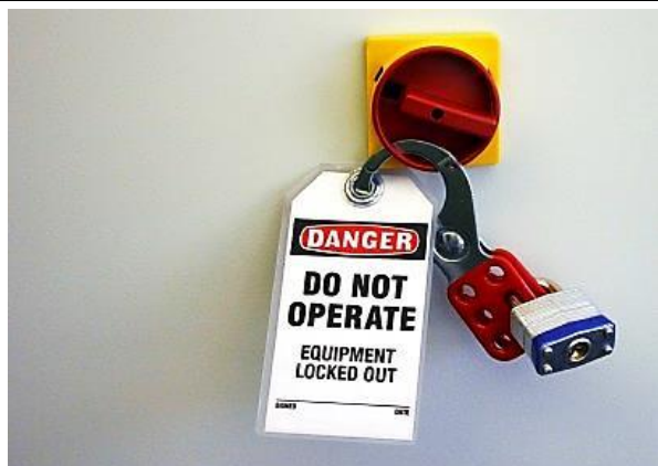
Equipment must be safely isolated and locked out prior to commencing trouble shooting, maintenance and repair activities
