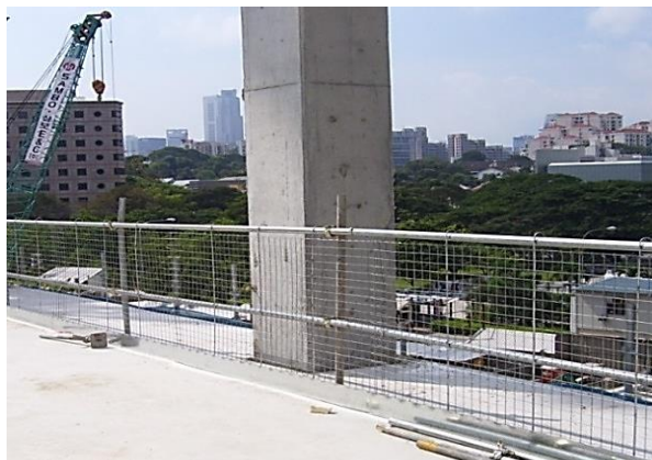
Rigid barriers with steel mesh are bolted onto the ground and set back to prevent equipment from being driven off the edge -
