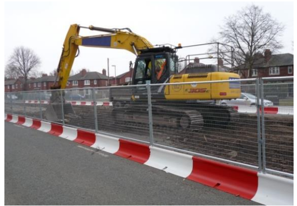
Barriers to prevent contact with pedestrian and vehicles
