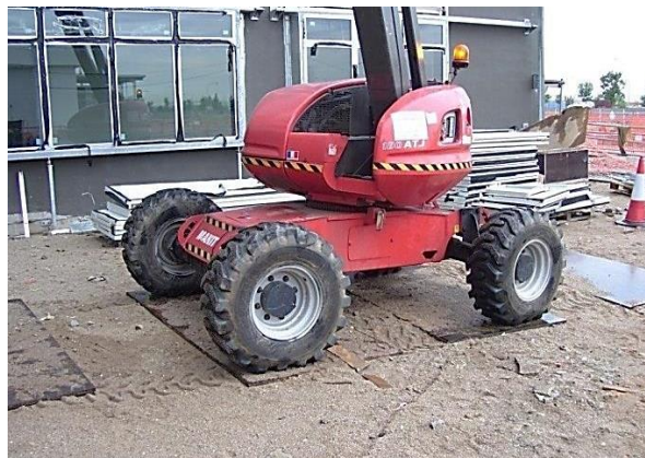
Engineered-approved steel plates provide stability during plant operation
