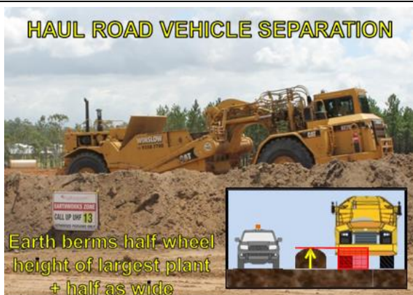
Segregation between light and heavy vehicles
