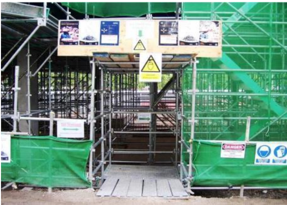
Overhead protection at designated access point of the building
