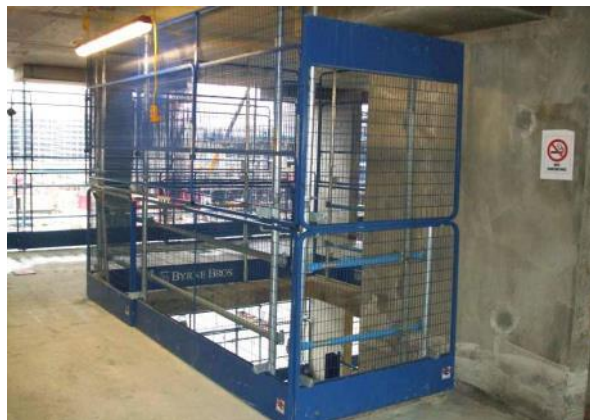
Large penetration protected with full height robust fence
