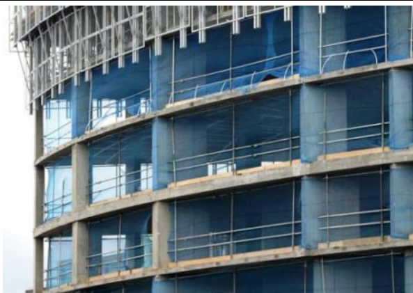
2 perimeter rails (top @ 1200mm and mid-rail @ half the height between top rail and toe boards), floor to soffit netting
