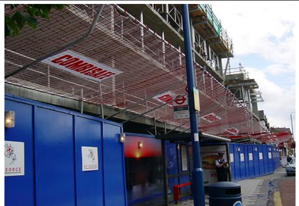
Safety net for fall protection for personnel
